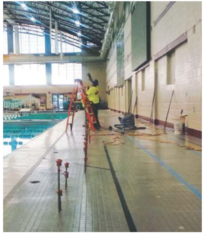
URETEK crews installed injection tubes in the pool deck at the Jim McKay Natatorium
