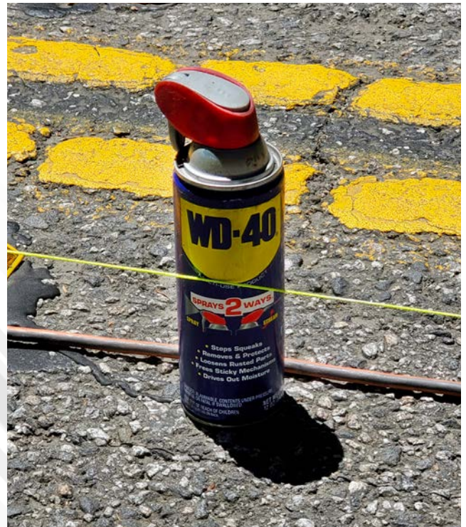
Clear pavement settlement was seen at the Boulder Creek job site
