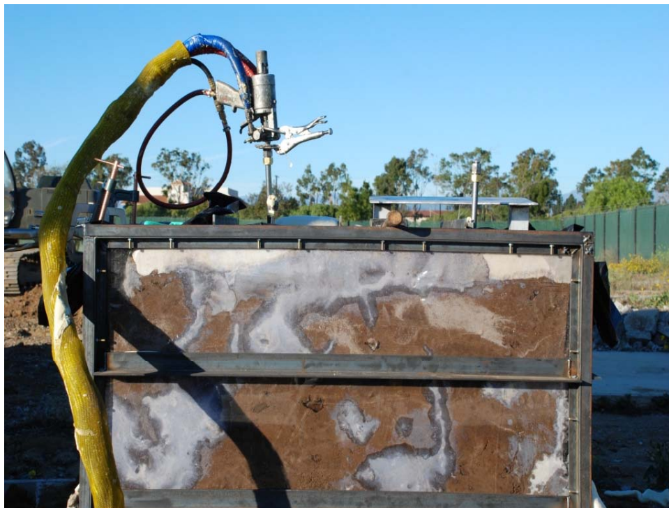
Injection inside steel reinforced, plexi-glass box so material flow could be observed
