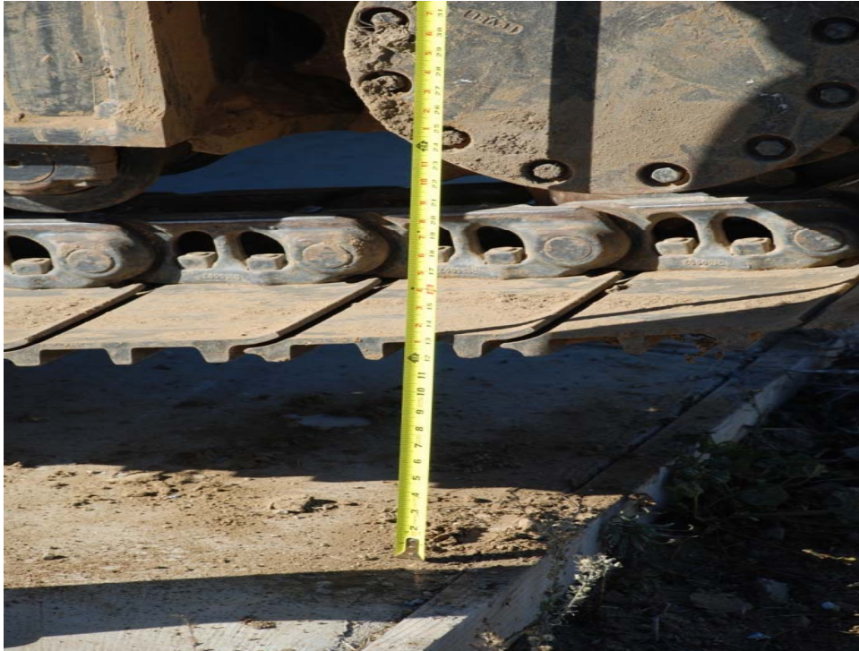
Soil mass would not crush, but excavator was lifted 11 inches
